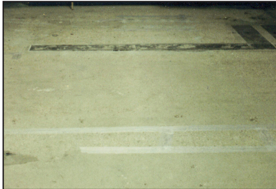
Exposed aggregate caused concern for paper contamination and operator safety
